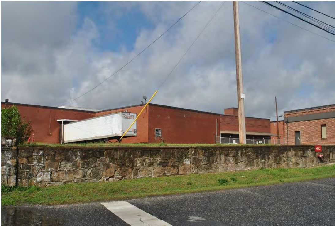
Groves Mills, Stone Retaining Wall on Grover Street, Looking Northwest Towards Mill No. 1.
