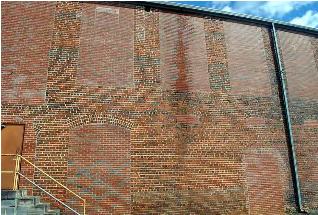
Seminole Mills, 1029 South Marietta Street, Gastonia, Infilled Window Openings.
