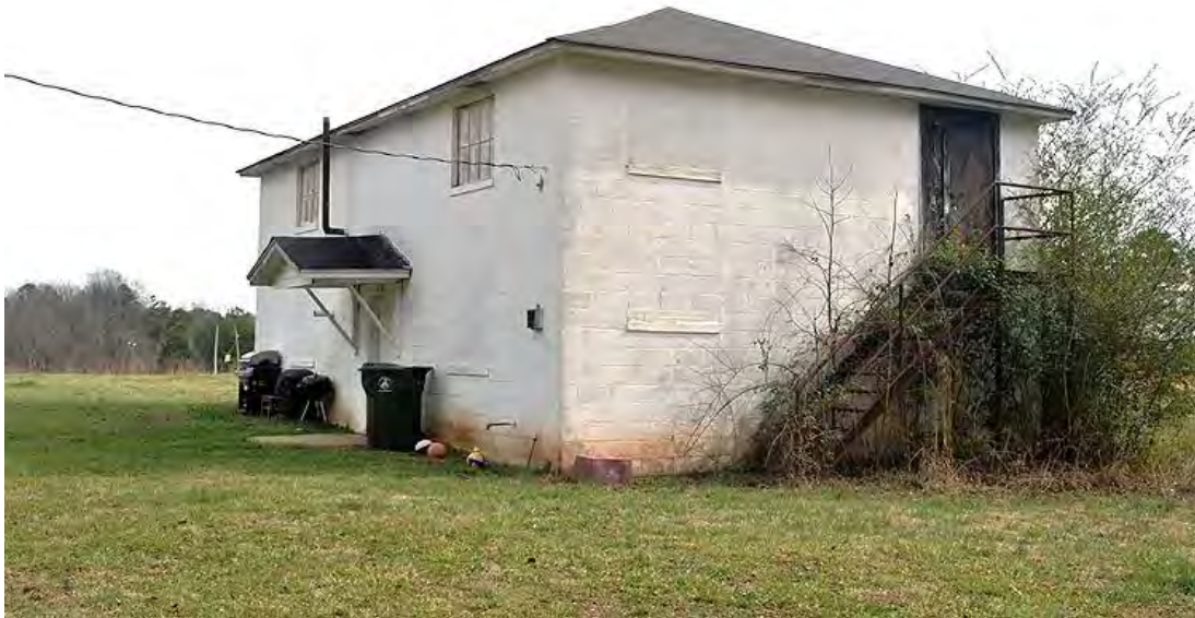
Hiram Masonic Lodge No. 22, Façade (North) and Side (West) Elevations, Looking East.
