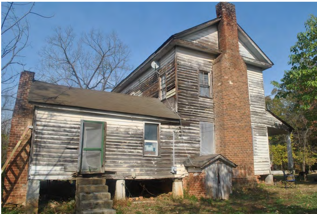
Caleb John Lineberger House, Side (South) Elevation and Rear Ell, Looking North.
