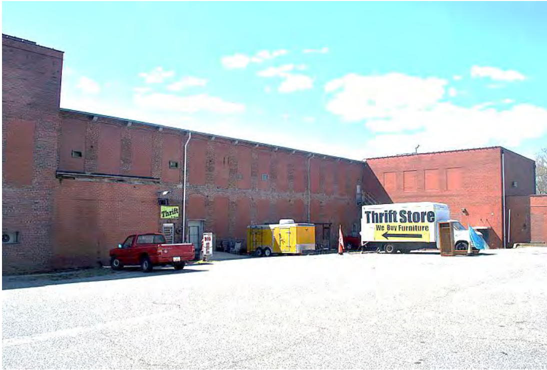
Modena Cotton Mills, Mill No. 2, Side (North) Elevation (1905) and Picker Room Addition (1940s), Looking West.
