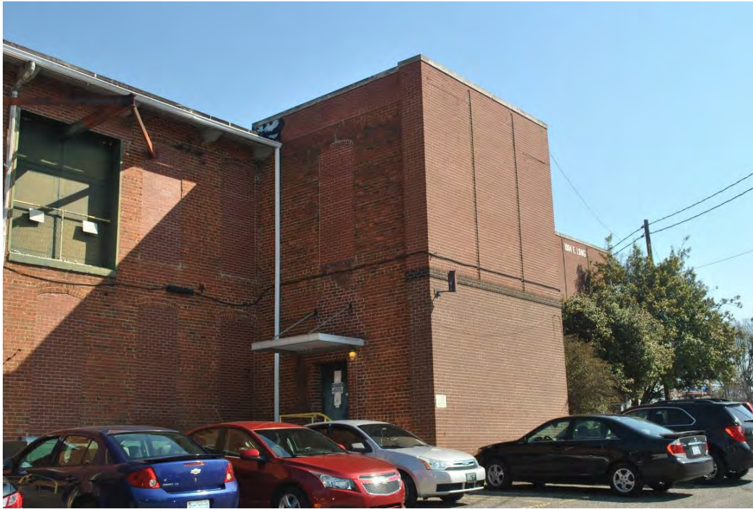
Modena Cotton Mills, Mill No. 1, 1894 Side (South) Elevation and circa 1965 Brick Veneer, Looking Northeast.
