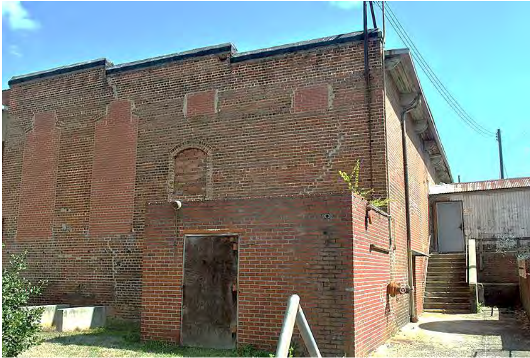
Modena Cotton Mills, Mill No. 2, Rear (West) and Side (South) Elevations (1905), Looking East.
