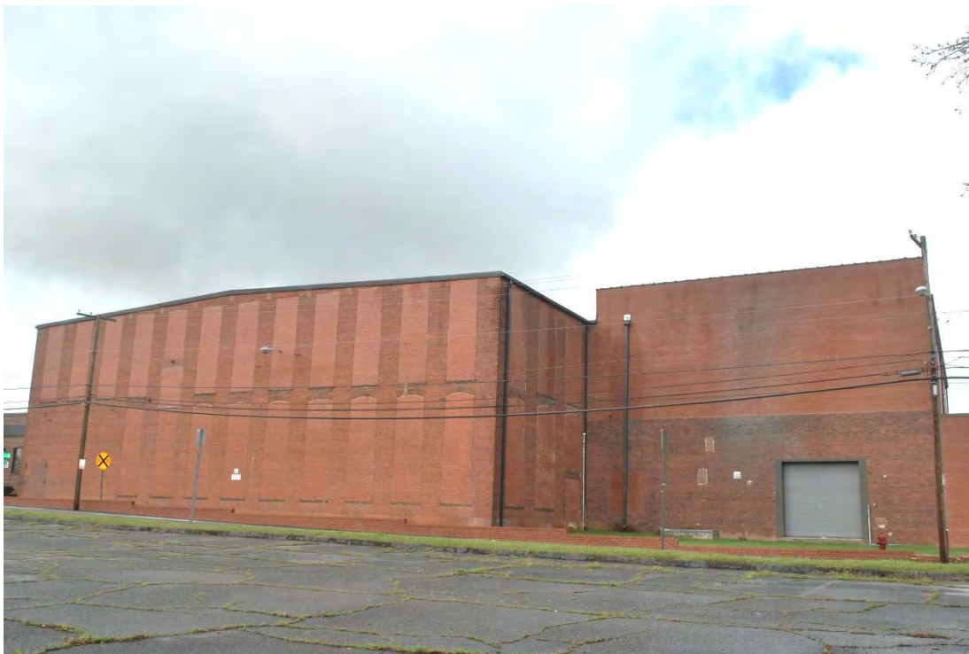
Groves Mills, Mill Nos. 2, and 3, East Elevations, Looking West from Grover Street,
