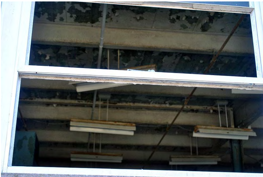
Hinde and Dauch Paper Company Factory, Office Interior, Showing Steel I-beam Structure.
