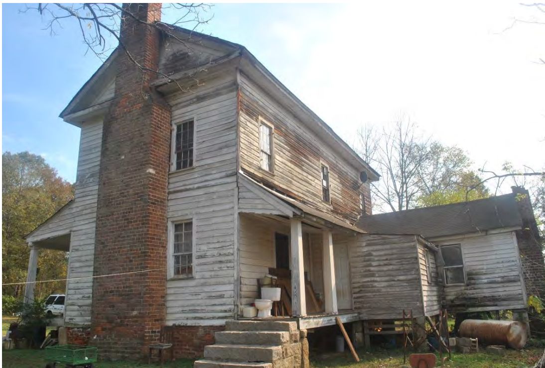
Caleb John Lineberger House, Side (North) and Rear (West) Elevations, Looking South.
